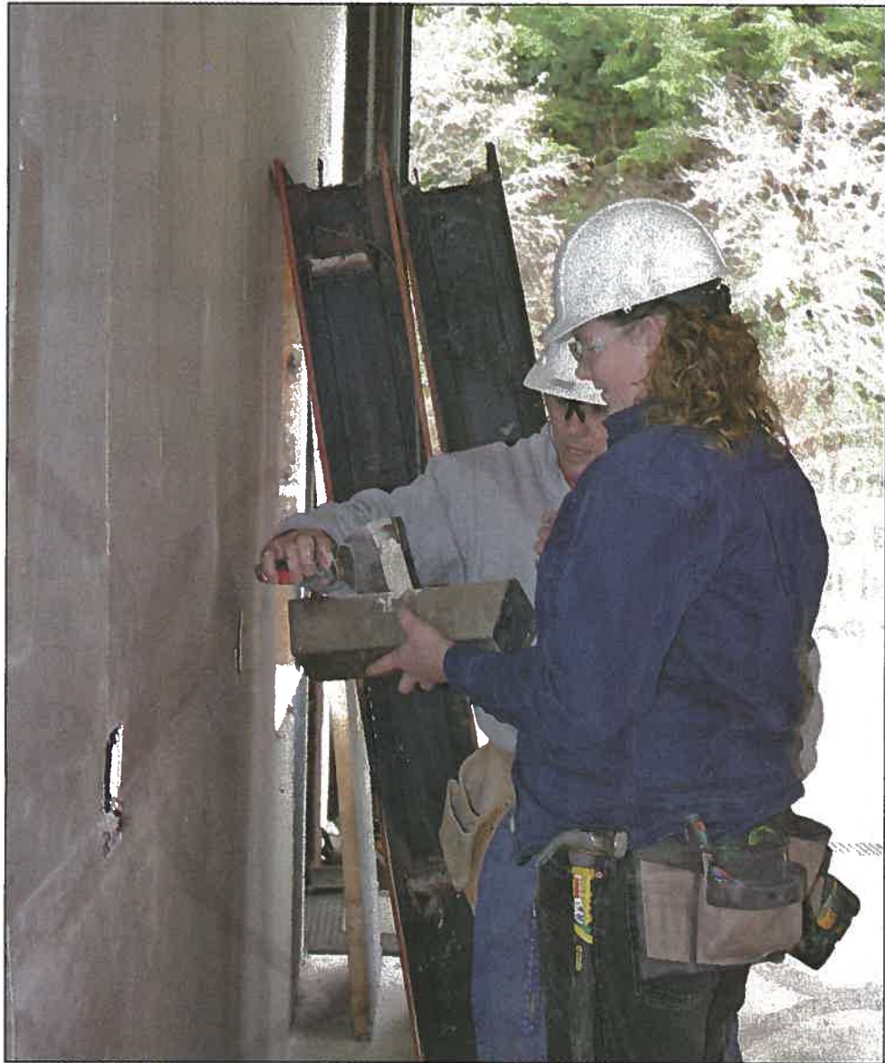
CSC youth work crew leader Peter Lohonyay shows Ashley DeVries how to apply plaster on sheetrock. DeVries is a member of the youth work crew team who worked on the old Toledo Fire Hall. Youth work crew members receive training and learn job skills while earning minimum wage. (Photos by Monique Cohen)
