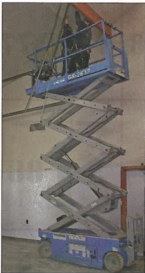
Frank Aguilar and Remington Iverson, members of the CSC youth work crew, are on the manlift installing sheetrock on the ceiling of
